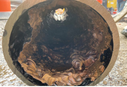
Mineral build-up over the years can cause water quality issues and trigger customer complaints
